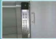
Elevator Control System
